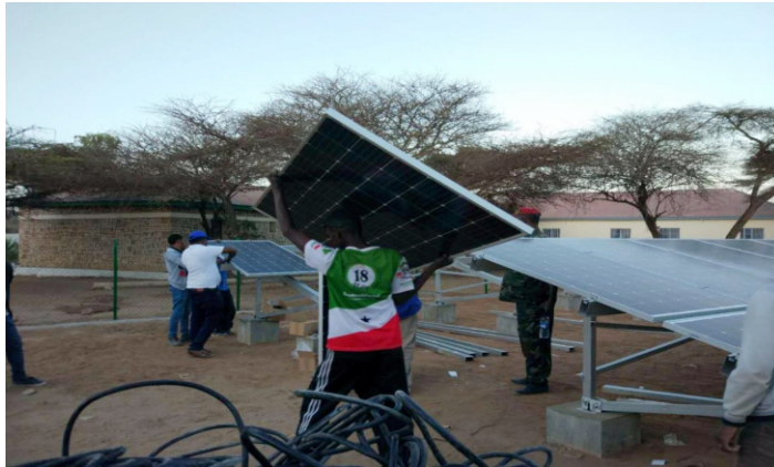
Army Hospital : 20KW Solar Off Grid System
