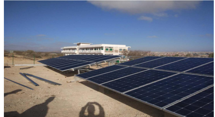
Army Head Quarter: 35KW Solar Off Grid System
